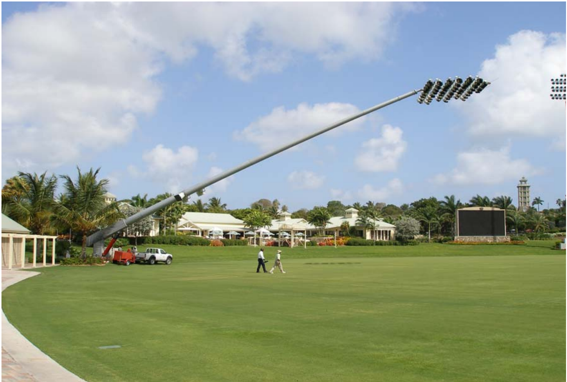
Field Flood Lighting
